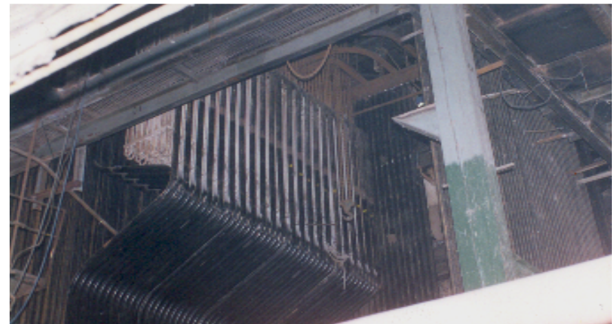
Boiler Tube Panel Erection, at: - M/s. U. P. State Sugar Corporation, Doiwala
